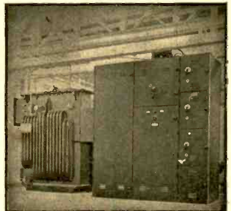
Sealed ignitron rectifier of factory-assembled load-center unit-substation type, installed in a large war plant. 300-kw, 250-v size.
